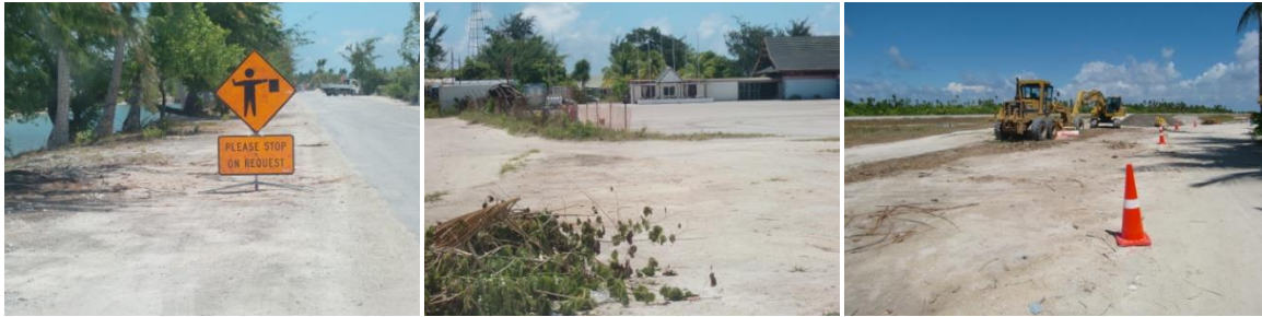
(1) public are learning about road signs; (2) some part of road behind Bonriki police cleared and widened with soak pit; (3) clearing at lagoon side of terminal at south-western end (photos by Temakei Tebano)
