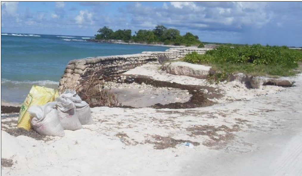
Figure 8 Seawall at north eastern end of runway showing erosion and bags of collected sand
